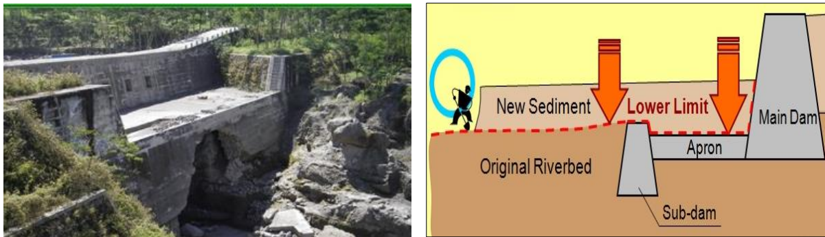
Figure 5. Eroded Sabodam (left) and Mining Limits (right) (Sumber: Jcpoweryogyakarta.Blogspot.Com)
